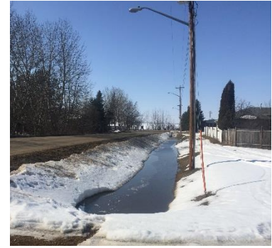
Ponding in ditch network (March 2019)
