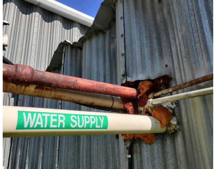
Figure 4-40: Ice Plant Room Pipe Penetrations
