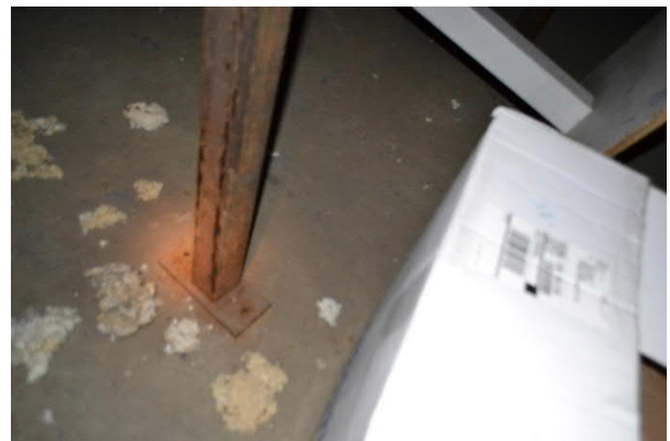
Figure 3-29: Base of Bleachers with Post & Baseplate Missing Bolts
