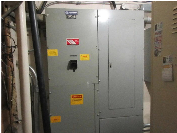
Figure 5-3: Main Distribution Panel - 800A, 120/208V, 3P, 4W
