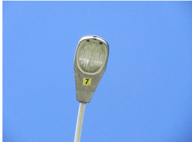
Figure 5-18: Typical HID Lighting Standard
