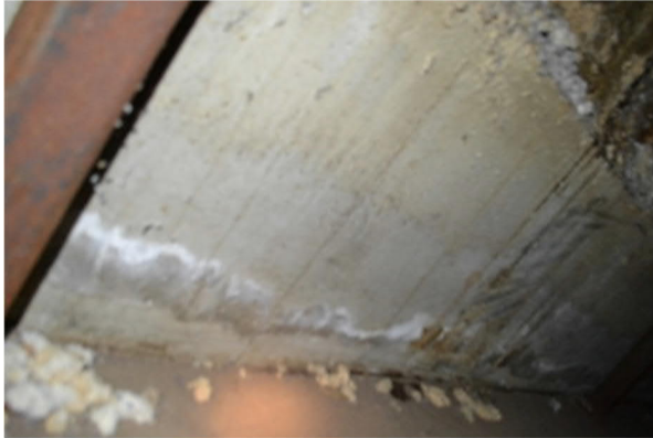
Figure 3-15: White Residue on Concrete Foundation Under Bleachers
