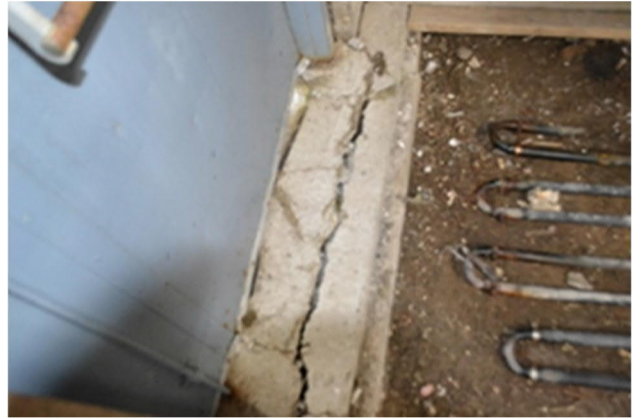
Figure 3-24: Severely Cracked Slab Thickening at Main Entrance
