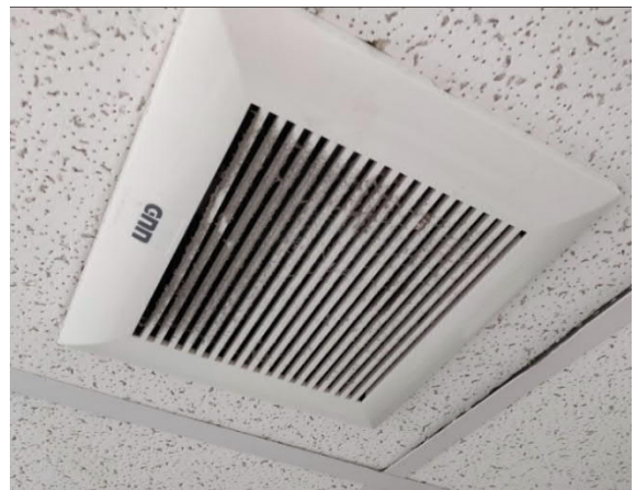
Figure 4-49: Typical Dust Buildup on Main Floor Exhaust Grilles
