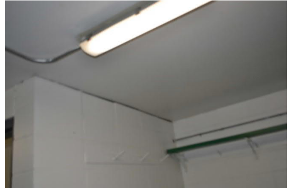
Figure 3-34: A Gap Between Ceiling & Masonry Wall
