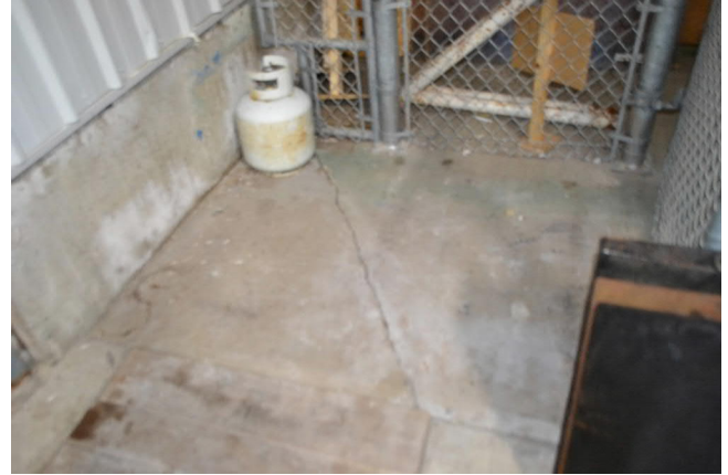
Figure 3-31: Cracked Plant Room Floor Slab
