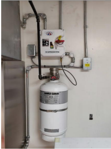
Figure 4-56: Fire Suppression Equipment Serving Kitchen Hood
