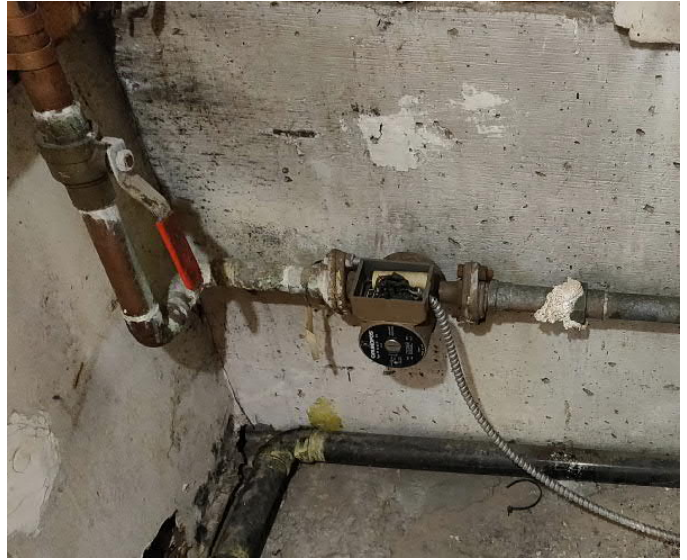
Figure 4-5: Significant Corrosion on Hot Water Piping
