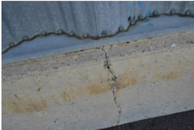
Figure 3-17: Shrinkage Crack on Building Foundation Walls
