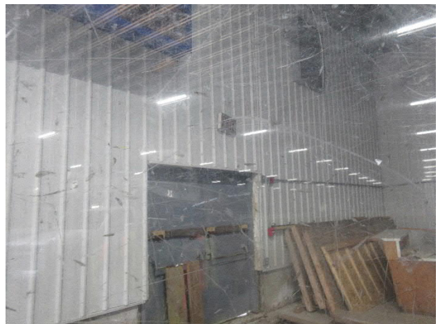
Figure 5-24: Broken Exit Sign
