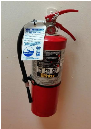
Figure 4-54: Typical ABC Fire Extinguisher on Wall Hook
