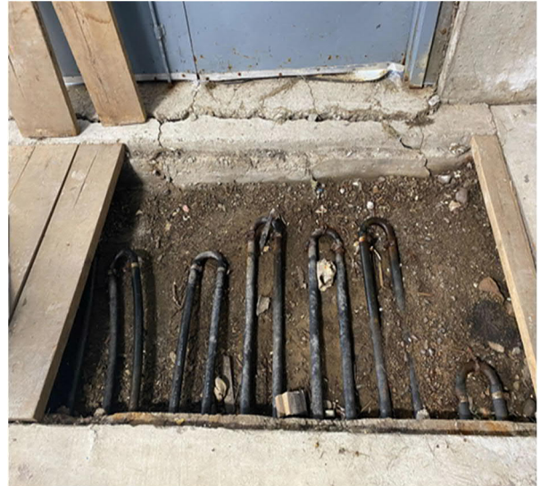
Figure 2-19: Ice Rink Tubes in Slab by Cracked Slab at Door
