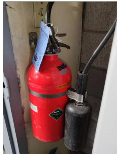
Figure 4-55: CO 2 Fire Extinguisher in Electrical Room
