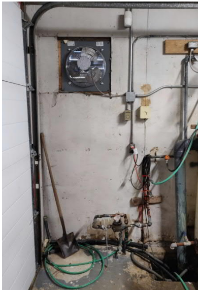
Figure 4-37: Ice Plant Room Ventilation Fan
