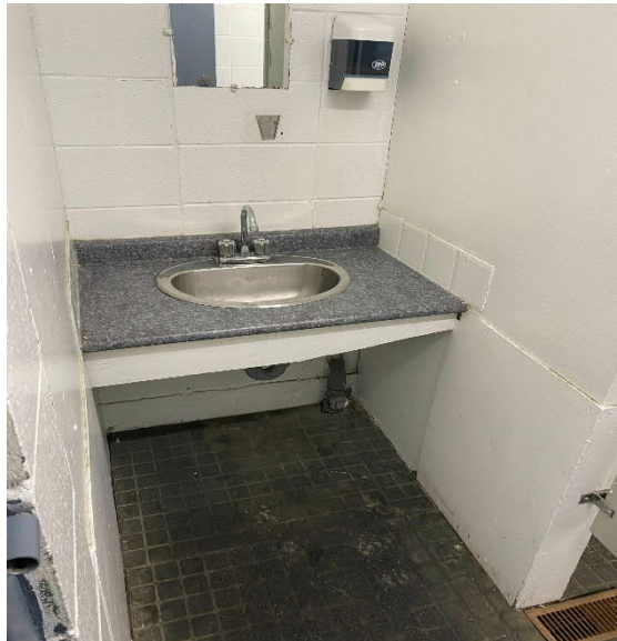
Figure 2-33: Typical Change Room Sink
