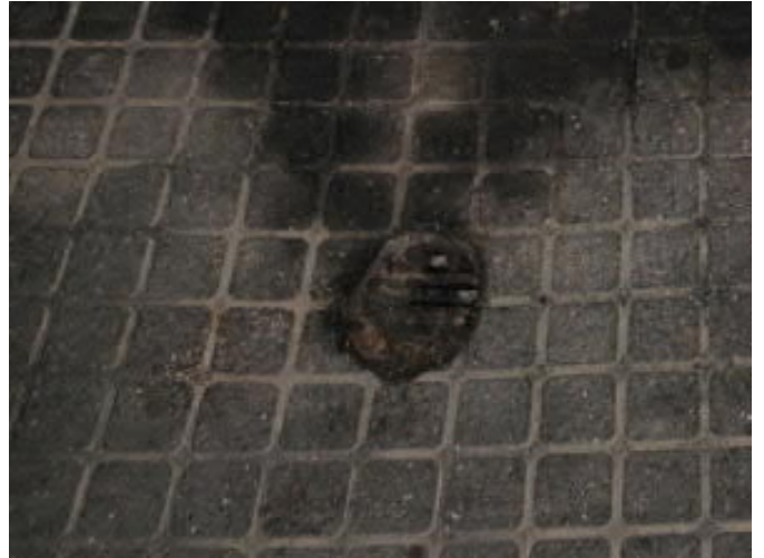
Figure 4-15: Typical Floor Drain on Main Floor
