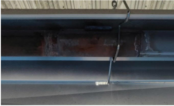
Figure 4-31: Corrosion on Tube Heater Surface
