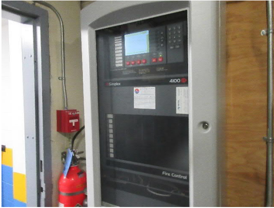
Figure 5-13: Main Fire Alarm Control Panel in Electrical Room
