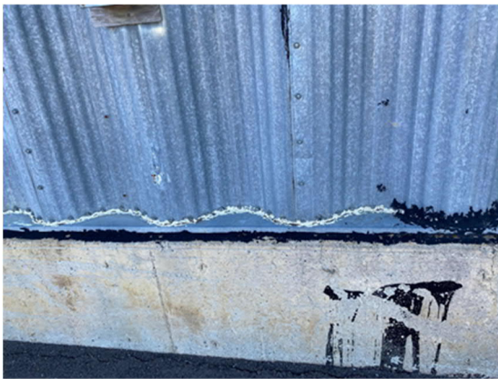
Figure 2-15: Caulking at Base of Metal Panel on West Facade
