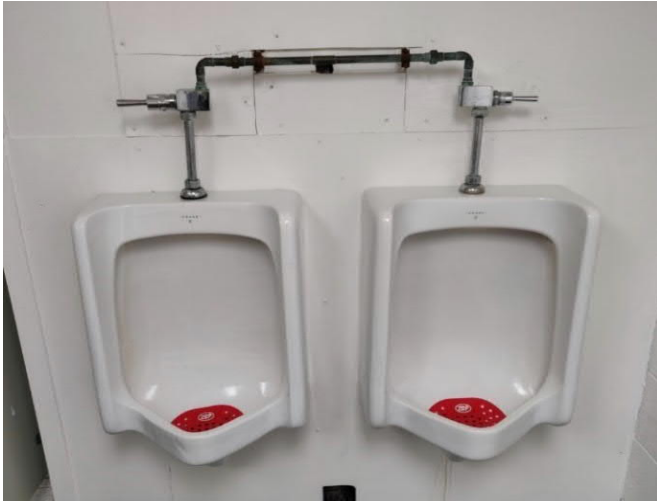
Figure 4-14: Mens Washroom Urinals
