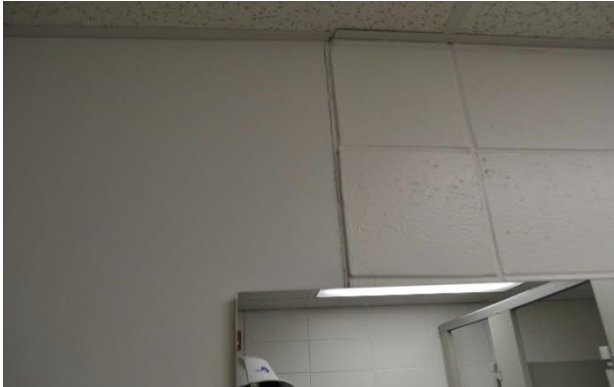
Figure 3-33: Crack Between Masonry Wall & Concrete Wall
