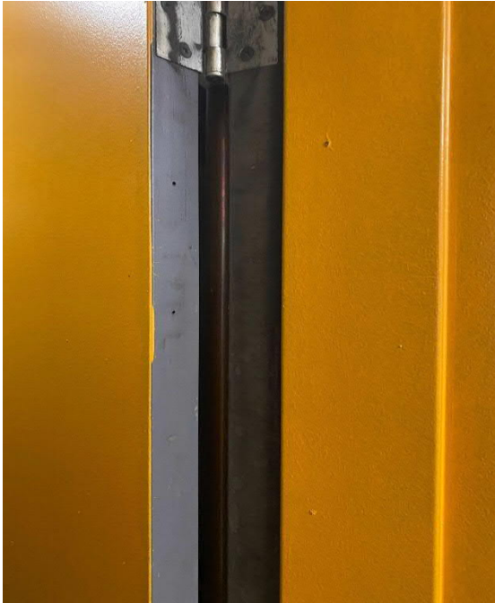
Figure 2-1: Door into Mechanical Room - Rating Missing
