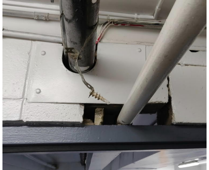
Figure 4-26: Damaged & Inadequate Pipe Hangers
