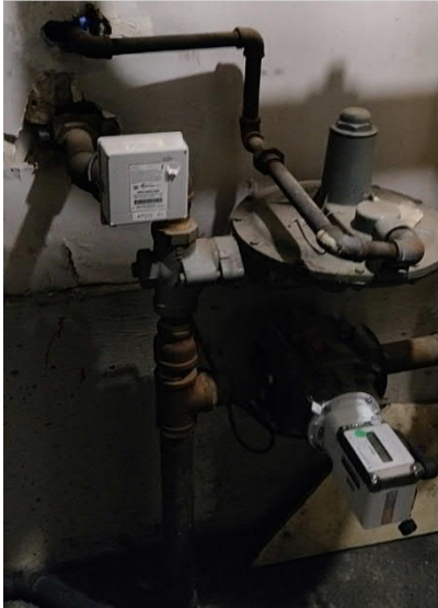
Figure 4-25: Gas Meter & Regulator in Mechanical Room
