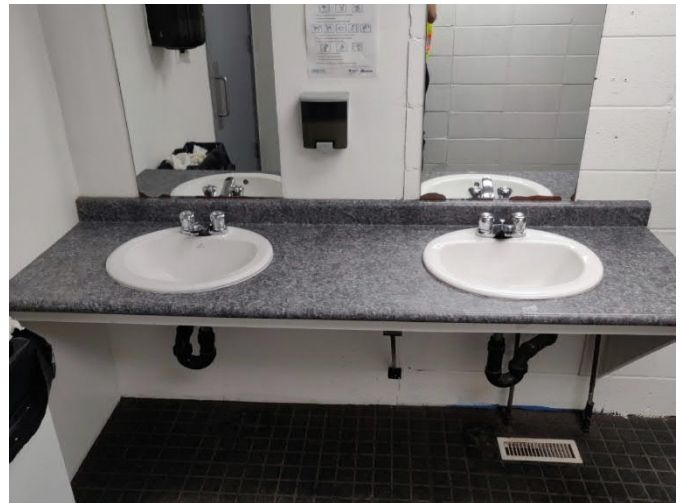
Figure 4-13: Typical Main Floor Washroom Lavatories
