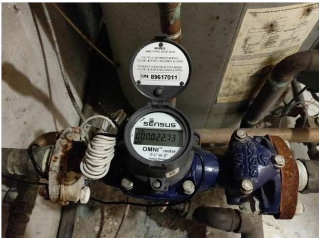
Figure 4-2: Building Water Meter
