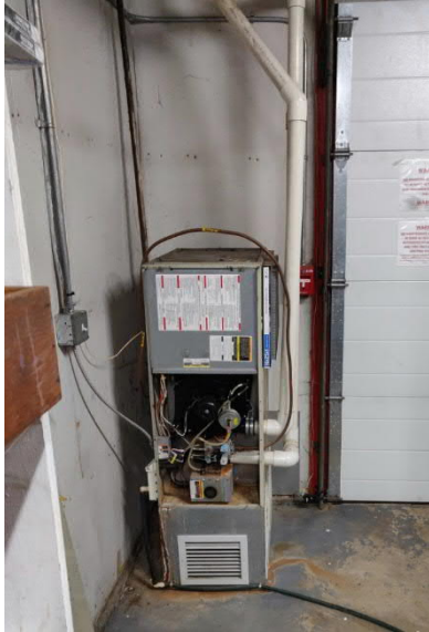
Figure 4-39: Ice Plant Room Furnace
