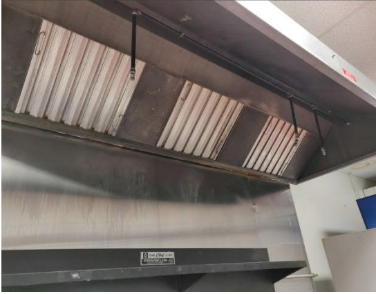
Figure 4-50: Kitchen Exhaust Hood
