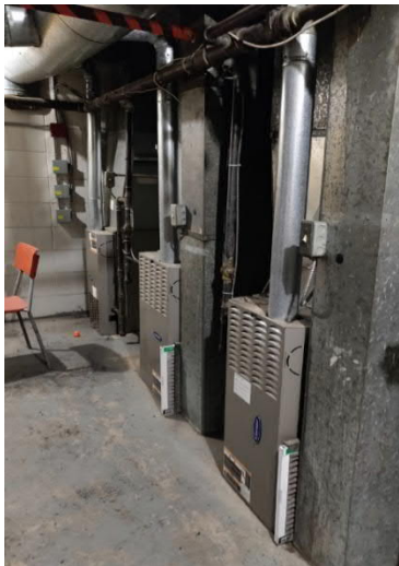
Figure 4-41: Furnaces Ventilating Building Areas
