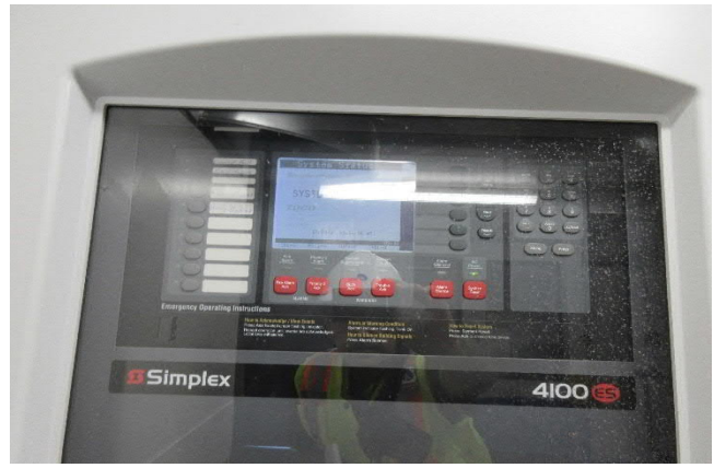
Figure 5-14: Main Fire Alarm Control Panel in Main Vestibule
