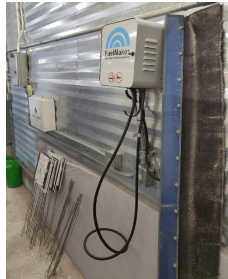
Figure 4-36: Zamboni Fuelling Station
