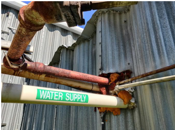
Figure 4-60: Heavily Corroded Piping to Outdoor Condensing Unit & Poorly Sealed Building Opening
