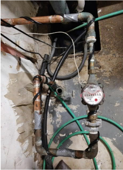
Figure 4-4: Ice Plant Water Entry & Meter
