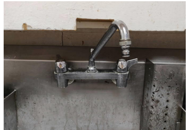
Figure 4-21: Kitchen Three-Compartment Sink Faucet
