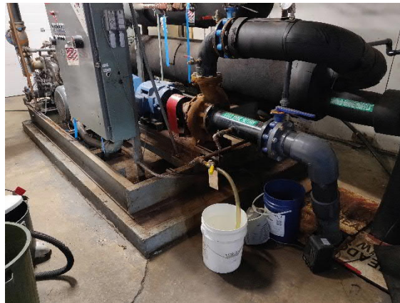
Figure 3-32: Ice Plant Room
