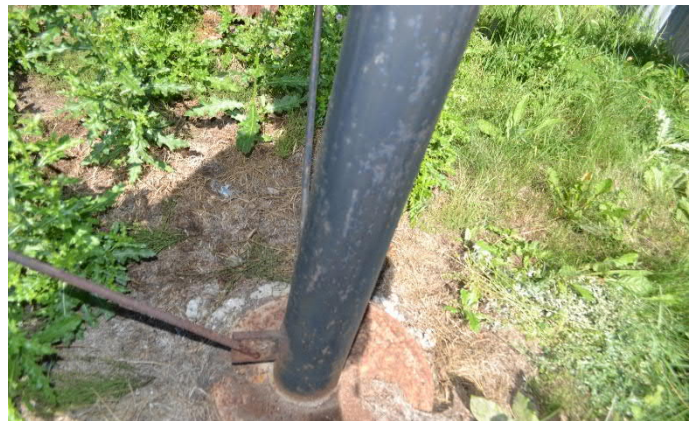
Figure 3-40: Rusty Base Plate
