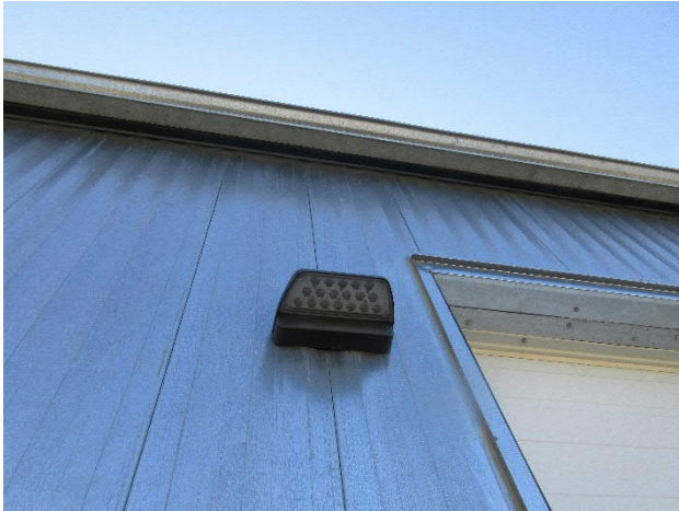
Figure 5-17: Typical LED Exterior Lighting
