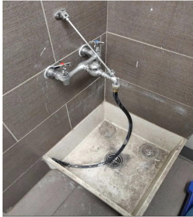
Figure 4-24: 2 nd Floor Janitor Room Mop Sink
