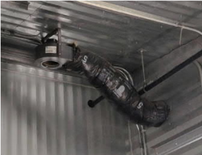
Figure 4-33: Zamboni Room Exhaust Blower
