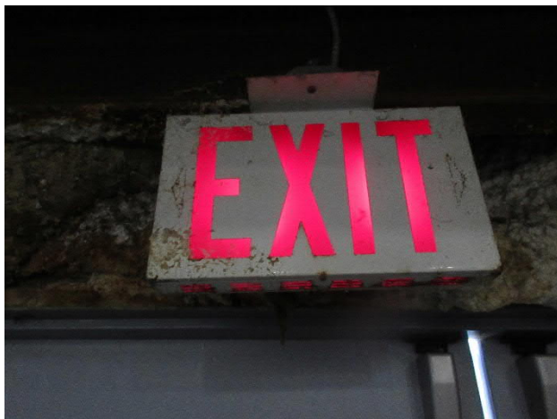
Figure 5-23: Rusty Exit Sign
