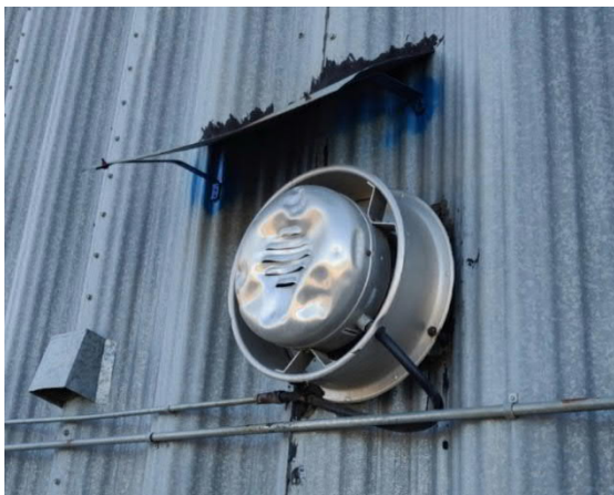
Figure 4-48: Locker Room Area Exhaust Fan
