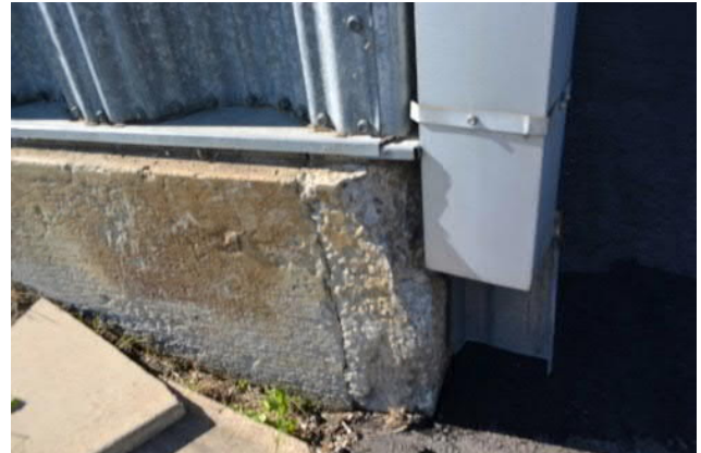
Figure 3-18: Concrete Scaling at Door Location
