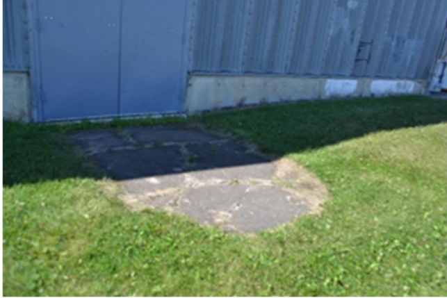
Figure 3-37: Deteriorated Exit Slab on North Side of Building
