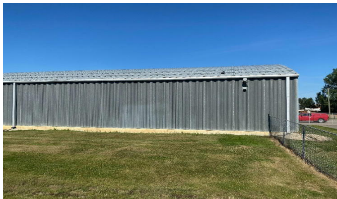
Figure 2-17: South Side – Rusting at the End of the Panels
