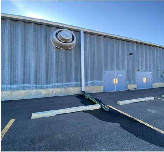
Figure 2-36: Drainage Issue on West Side
