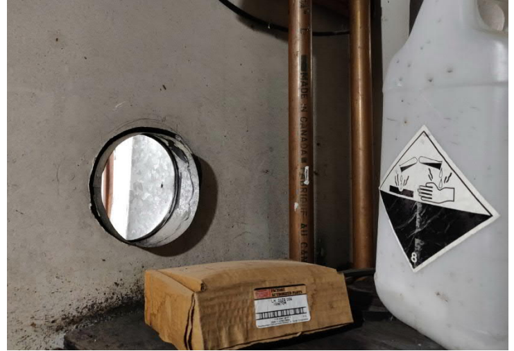
Figure 4-57: Opening in Mechanical Room Wall Without Fire Damper
