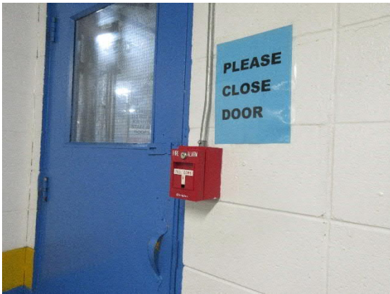
Figure 5-15: Typical Pull Station by Each Exit
