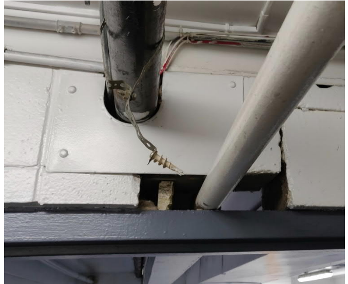
Figure 4-7: Damaged & Inadequate Pipe Hangers
