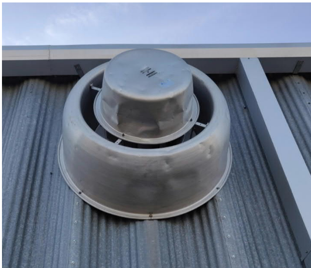
Figure 4-27: Typical Arena Exhaust Fan
