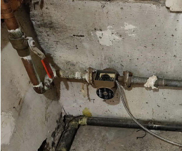
Figure 4-10: Domestic Hot Water Recirculation Pump in Mechanical Room
