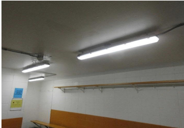
Figure 5-21: Dressing Room Lighting
