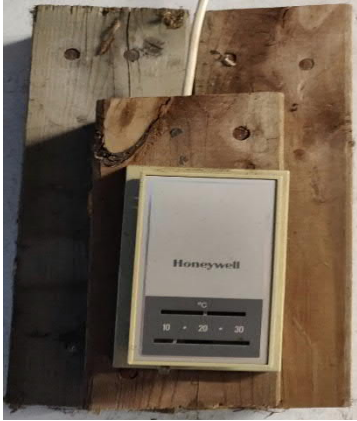
Figure 4-43: Typical Thermostat for Heating Equipment
