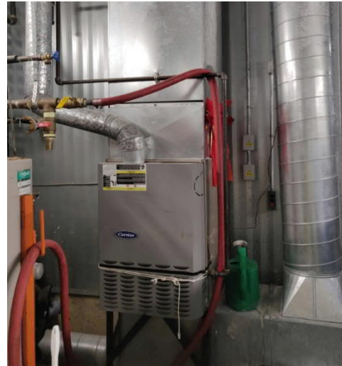
Figure 4-34: Zamboni Room Furnace &amp; Ductwork
