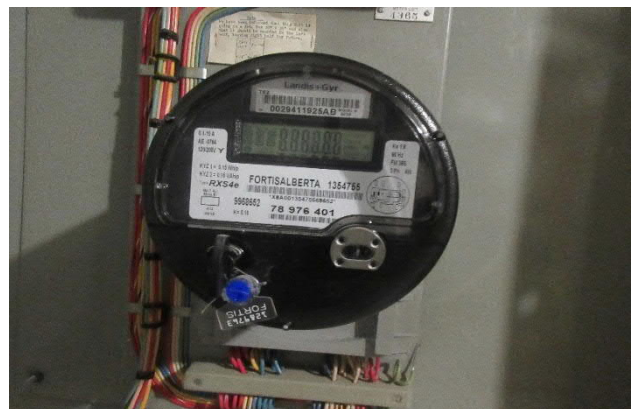
Figure 5-2: Indoor Utility Meter
