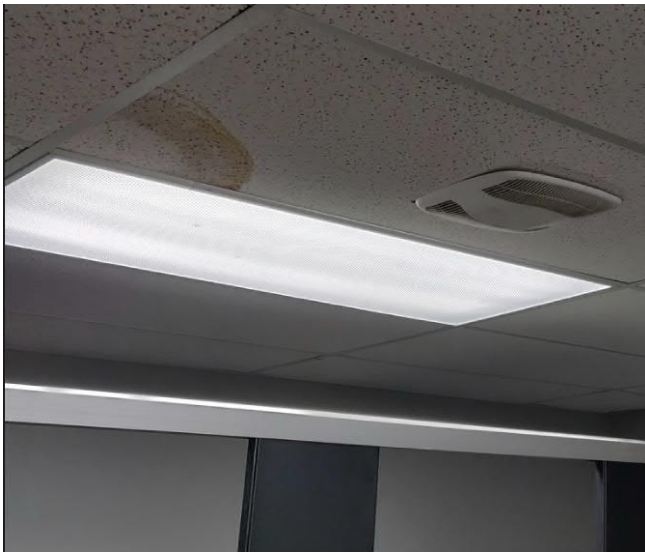
Figure 4-6: Ceiling Stain in 2 nd Floor Washroom
