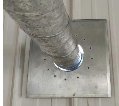
Figure 4-32: Poorly Sealed Tube Heater Flue Opening
