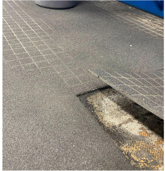
Figure 2-31: Skate Flooring Peeling Up with Gaps at the Corners
