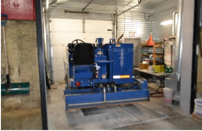
Figure 3-30: Plant Room Overview
