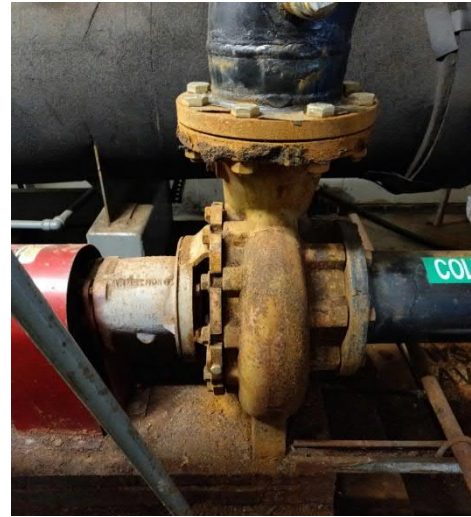
Figure 4-59: Significant Corrosion on Unprotected Pump Casing
