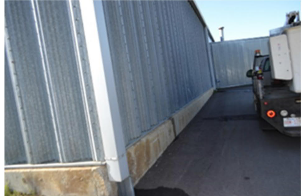
Figure 3-16: Concrete Discolouration of Foundation Wall Typical
