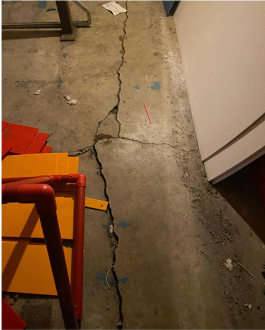
Figure 2-24: Crack in Slab on East Side of Rink under Bleachers
