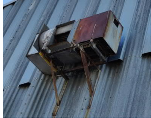
Figure 4-51: Kitchen Hood Exhaust Fan
