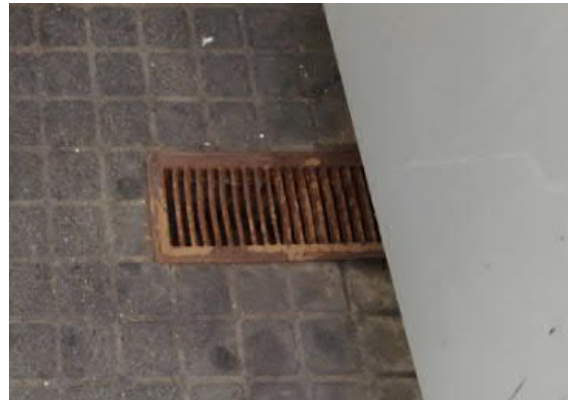
Figure 4-46: Typical Corroded Supply Grille in Locker Area Shower Room
