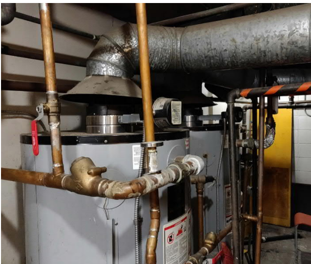
Figure 4-8: Water Heaters in Mechanical Room
