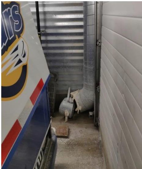
Figure 4-35: Damaged Air Terminal in Zamboni Room
