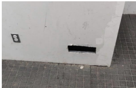
Figure 4-47: Typical Missing Ventilation Grille
