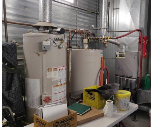
Figure 4-11: Domestic Hot Water Heater, Storage Tank & Circulation Pump in Zamboni Room
